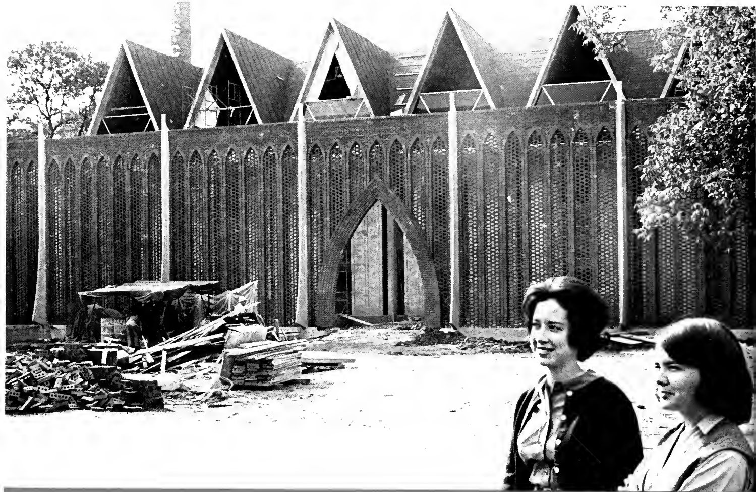
Beautiful weather this fall has kept construction of the Charles E. Dana Fine Arts Building right on schedule. The new building will be finished in January.
